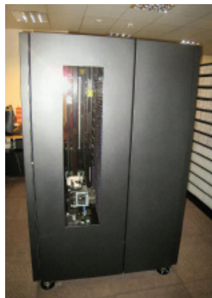
Figure 2 The IBM TS3500 ATL located in the DRS Building. The internal racking is visible and the robotic “hand” mechanism can be seen at the bottom of the cabinet. LTO tapes are also stacked on the external racking to the right of the ATL.
