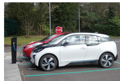
Charging points. ECMWF has installed two 16 A (3.6 kW) charging points free to use by staff and visitors at Shinfield Park.
